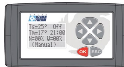
PIC 06: View of the control panel
